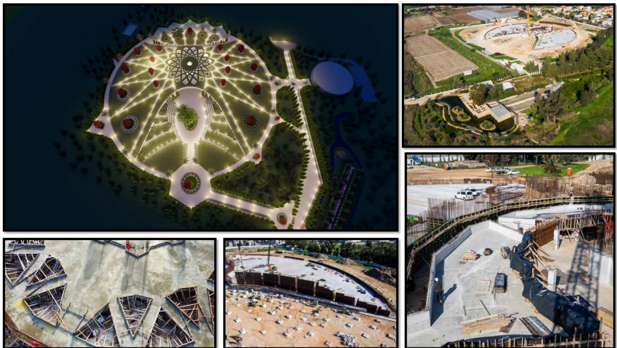
Some of the extraordinary progress that has been made on the construction of the Shrine of 'Abdu'l-Bahá (design, top left) in the past year, despite the various restrictions and limitations caused by the global health crisis.
