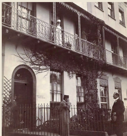
The restoration work on 17 Royal York Crescent, Bristol, where 'Abdu'l-Bahá stayed on two occasions, is well under way.
